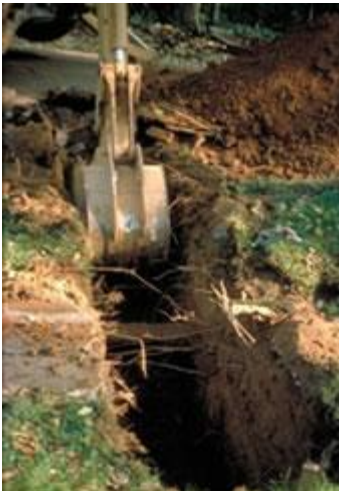
Figure 3. Backhoes digging utility trenches rip tree roots apart, exposing injured roots to infection by decay fungi.
