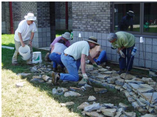
Participants of a dry stone workshop helped build a low retaining wall at Westridge Elementary
