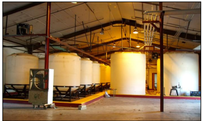
Pictured: Greearth Biofuels Plant, Kirkland Avenue, Irvine.
