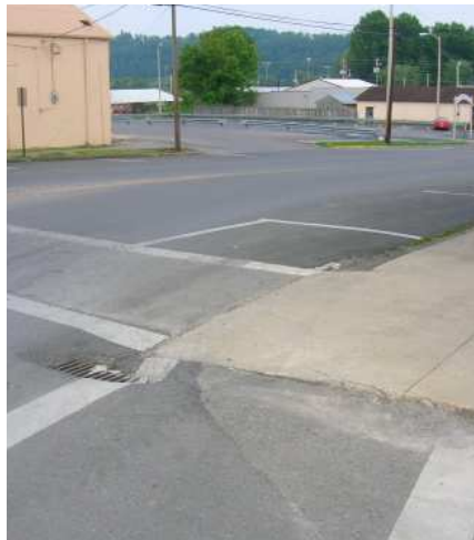
Existing curb ramps are inaccessible and poorly delineated.
