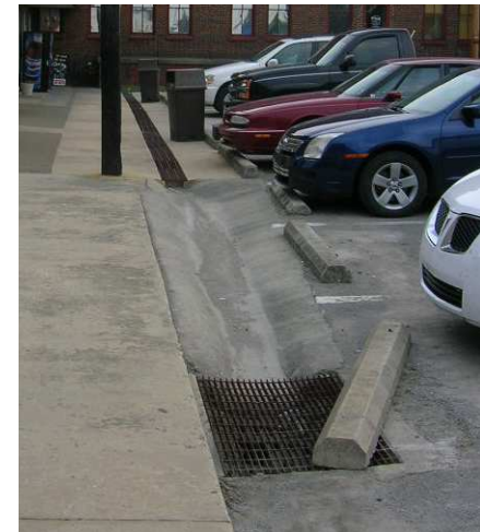
Existing stormwater management creates conflicts with pedestrian circulation as well as erosion issues throughout Main Street
