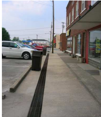
The current sidewalk condition suffers from lack of maintenance, utility poles and signage in the pedestrian environment, minimal projection between pedestrian and vehicle.
